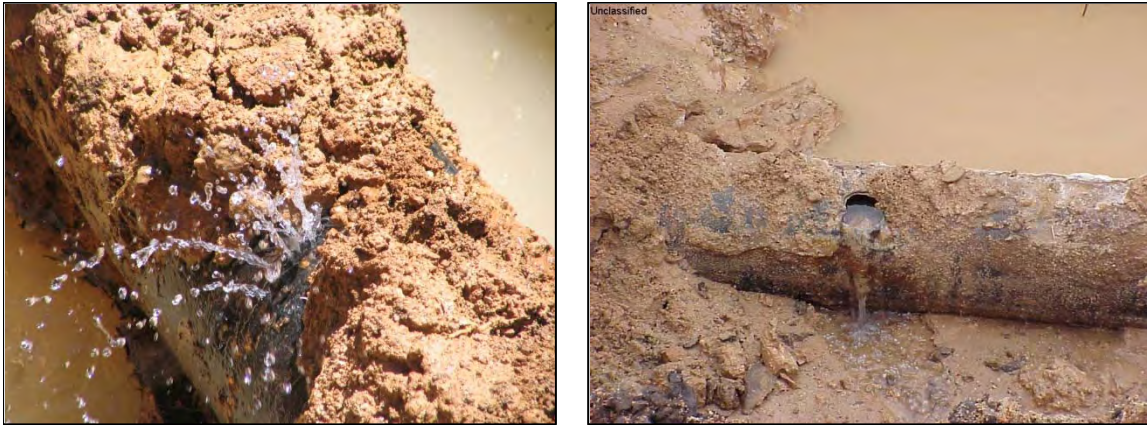
Figure D-16. Fire Protection Lead-In Piping Corrosion.
